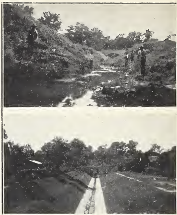
FIG. 1. Vicksburg, Mississippi. Upper, before malarial control drainage; lower, after construction of reinforced concrete invert with sodded banks.
